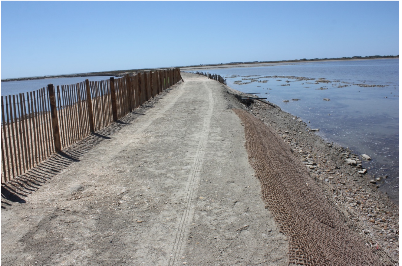
Figure 2 - Photo of the current progress of work (July 2020) of the DIGUE2020 platform
