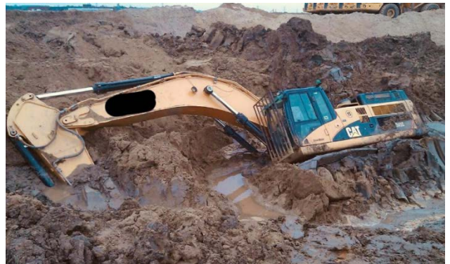
Figure 1 – Fallen machinery due to slope failure
